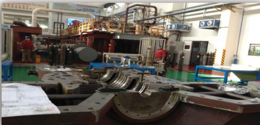
Syngas Compressors (LP/HP) c/w Mechanical Drive Steam Turbine
