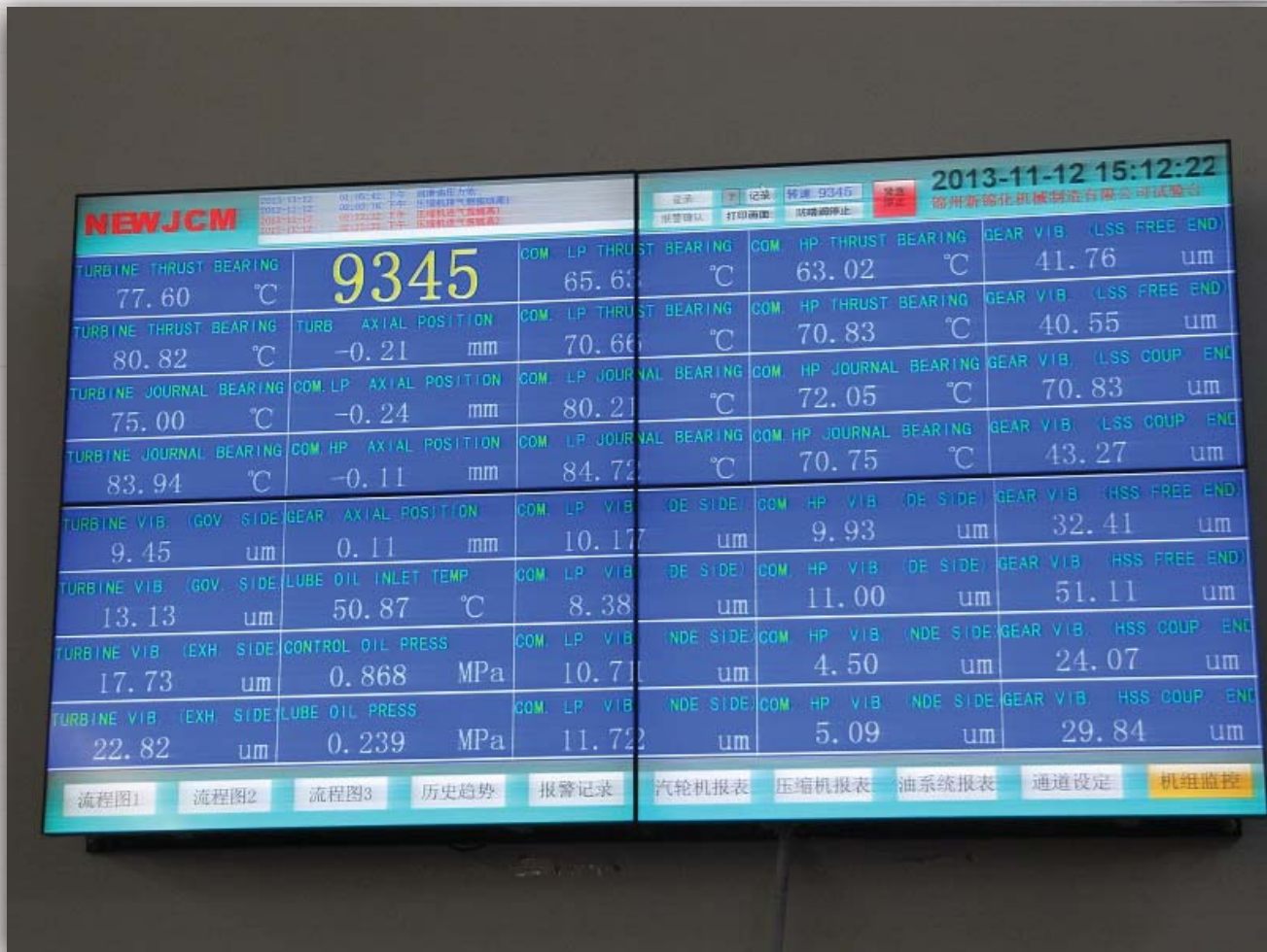
HMI Showing all important test data
