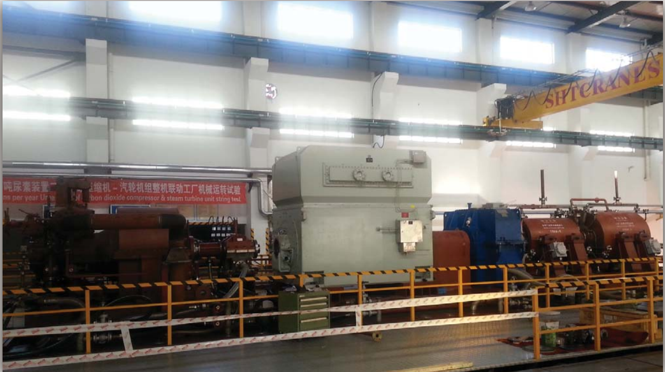
String Test of Complicate train: Including 6 equipment Steam turbine-Gearbox-VFD Motor-Gearbox-LP compressor –HP Compressor
