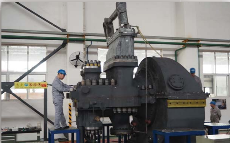
NEW JCM Technicians conducting assembly and inspection works for the MHI 40MW mechanical drive steam turbine for crack gas compressor.
