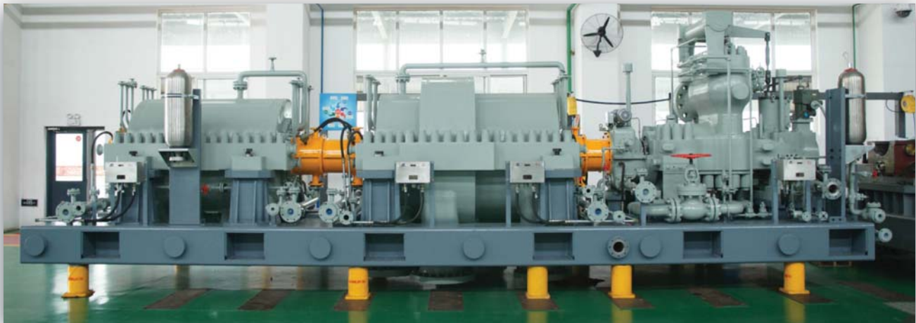
CO2 Compressors (LP/HP) c/w Mechanical Drive Steam Turbine
