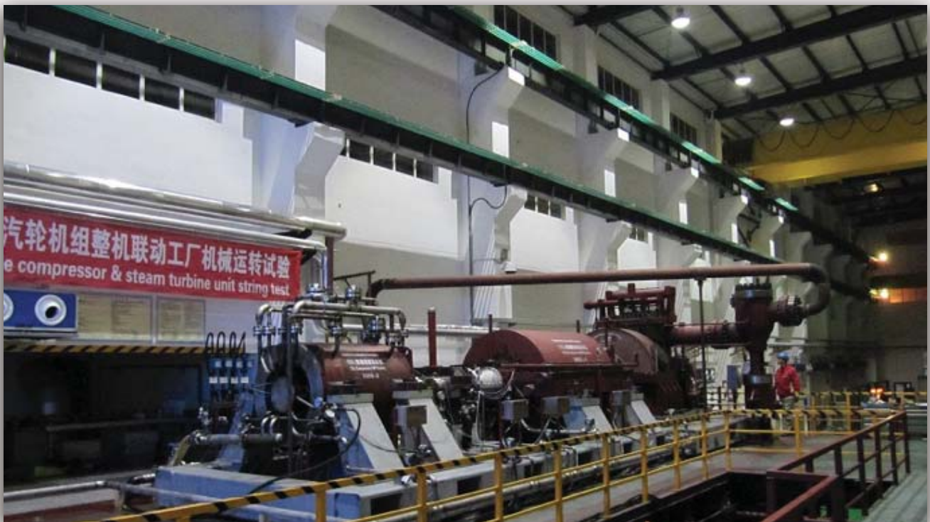
String Test of of CO2 Train: Steam Turbine – LP Compressor- Gearbox- HP Compressor
