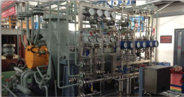
Sales Gas Compressors c/w Dry Gas Seal Control Panel on Skid
